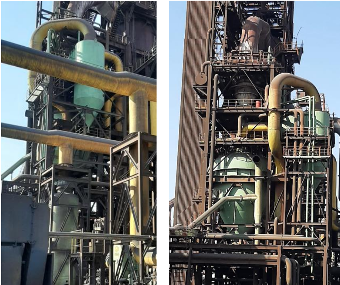
Fig.01 Top Gas Scrubber Cyclone Mist Eliminator
